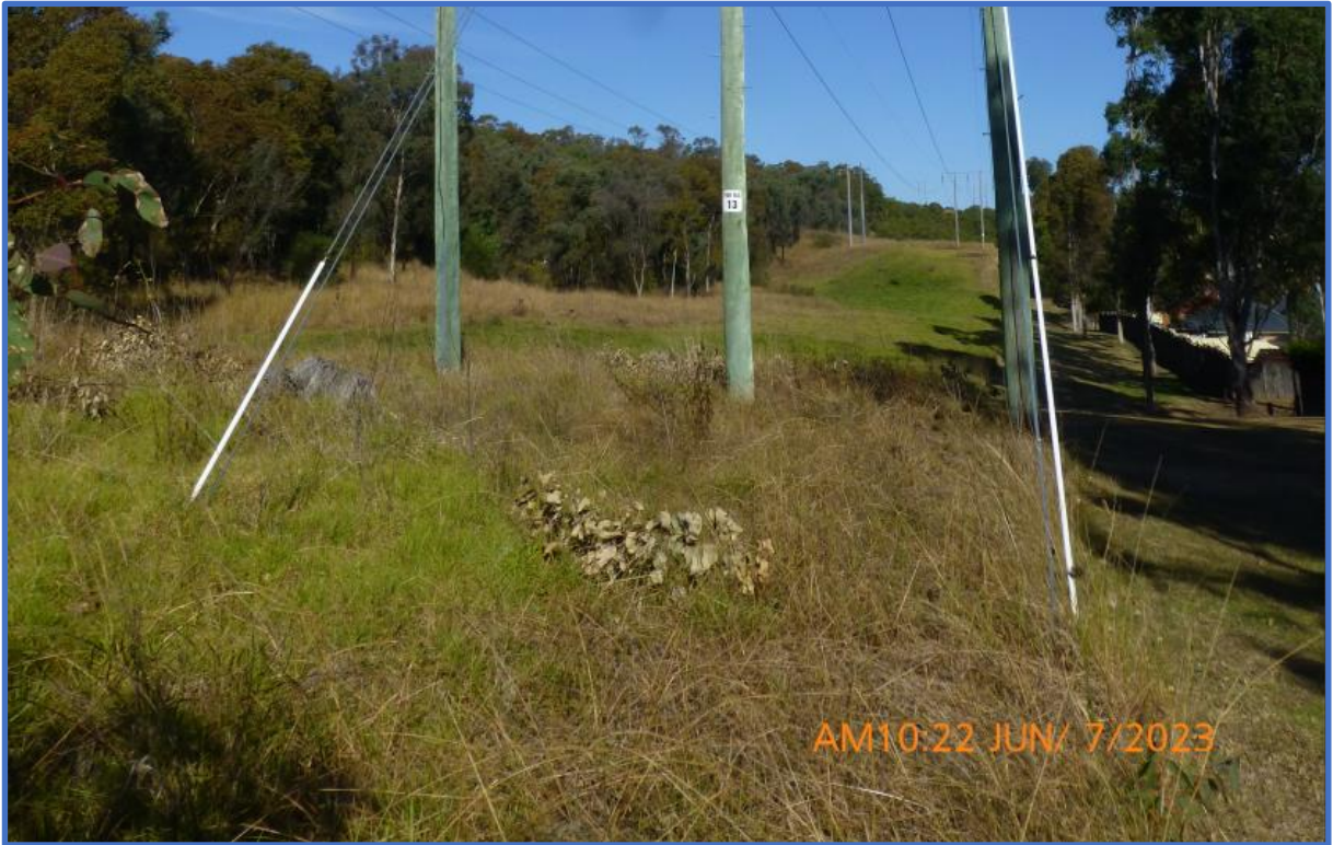
Figure 20: Ground surrounding Pole 13 to be replaced and new stays installed
