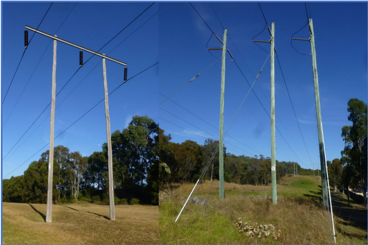
Figure 10: Examples of a H pole (left) and a 3-pole structure (right)
