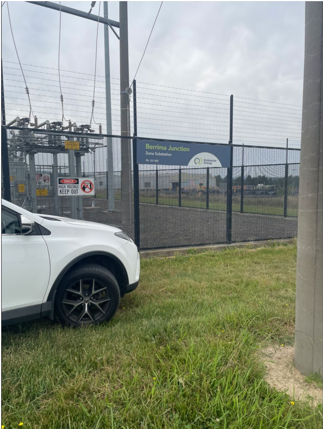
Plate 1. Current Berrima Junction Zone Substation
