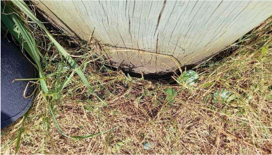
Plate 2.2 15 mm gap between pole 212270 and the ground
