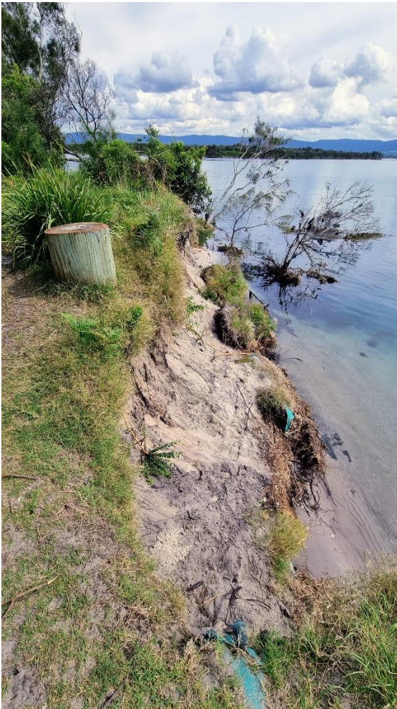
Plate 2.3 Stump of pole 212270
